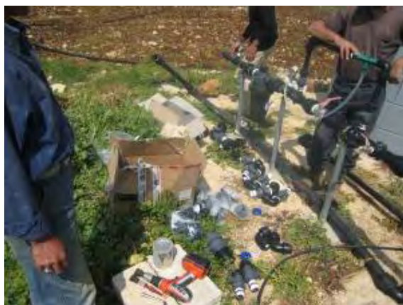
Figure 19. Installation of a fertigation unit including a ventury system and a disk filter
