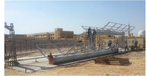
Trough Units at site
