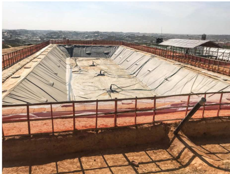
The human waste treatment facility under construction at the refugee settlement near Kutupalong, Bangladesh. © UNHCR/Firas Al-Khateeb
